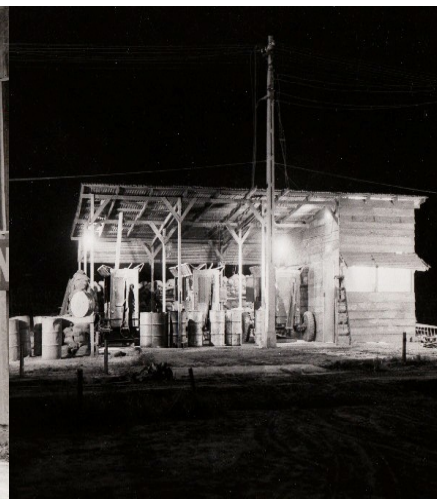
The three portable diesel generators maintained by the utilities section, ran day and night to provide the base with electrical
